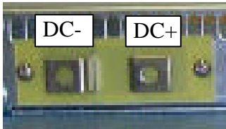
DC Input Buss Bars (cover removed)
